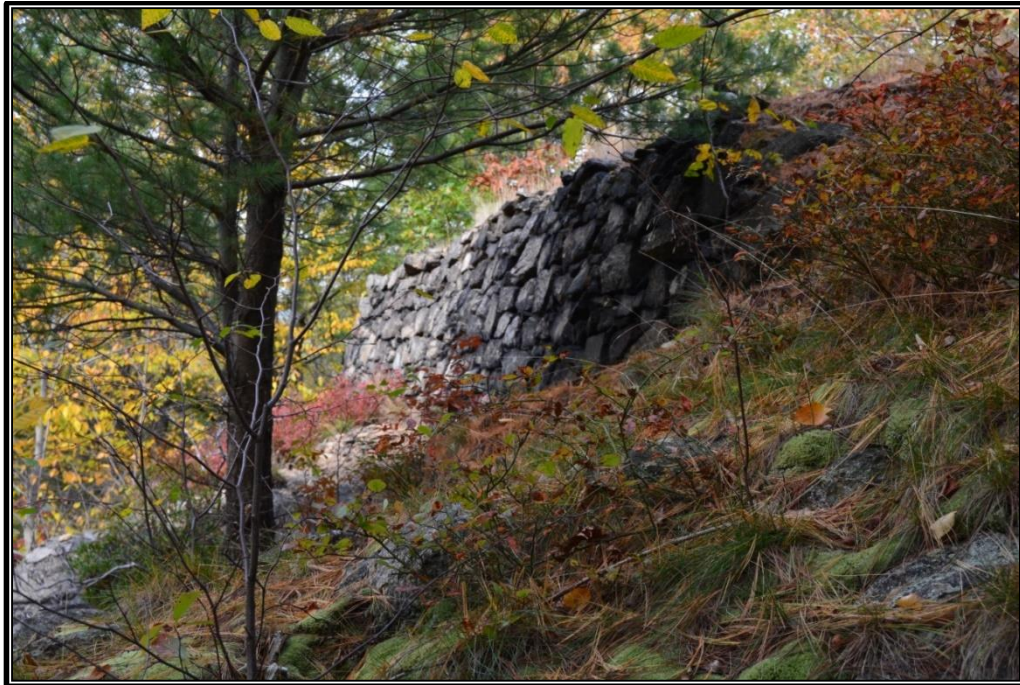
The northern portion of the west Redoubt 5 rampart, showing its stone revetment, facing north (Panamerican 2016).
