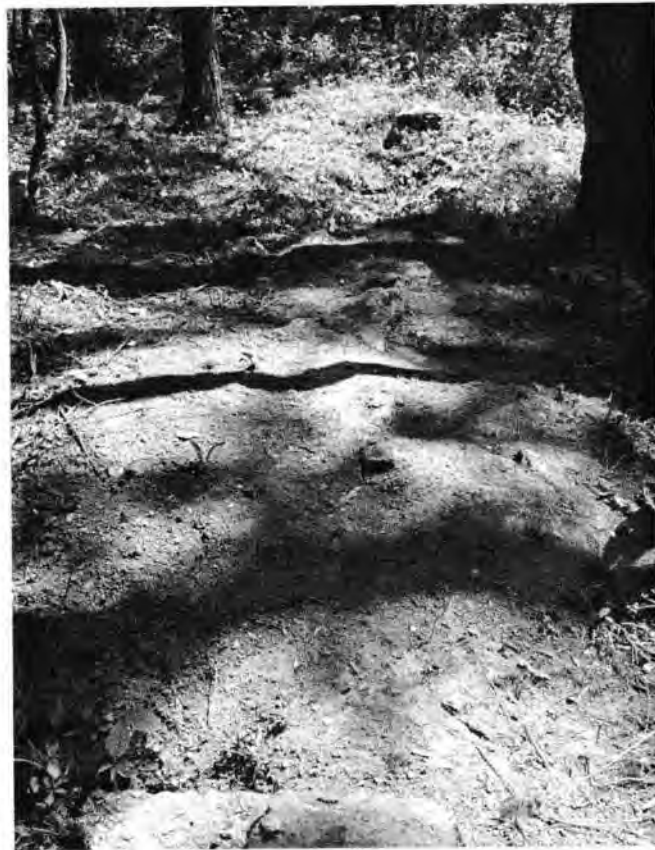
Figure 24. View looking south from the southwest corner of the Adams House foundation. The corner of the main foundation is located in the foreground and the remaining foundation stones for the addition are running south from the corner.
